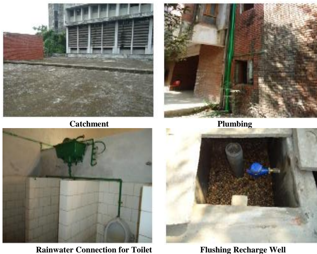
Figure 4: Rainwater Harvesting System of BUET
